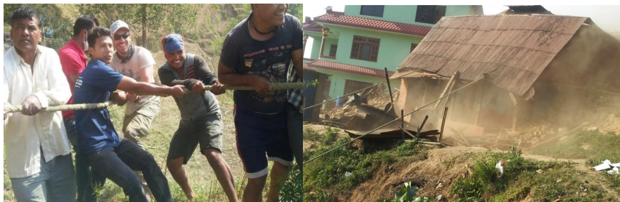
Figure 8 VIN's staff, volunteers and locals are working to demolish the cracked houses
